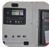
Control Panel & MCB
